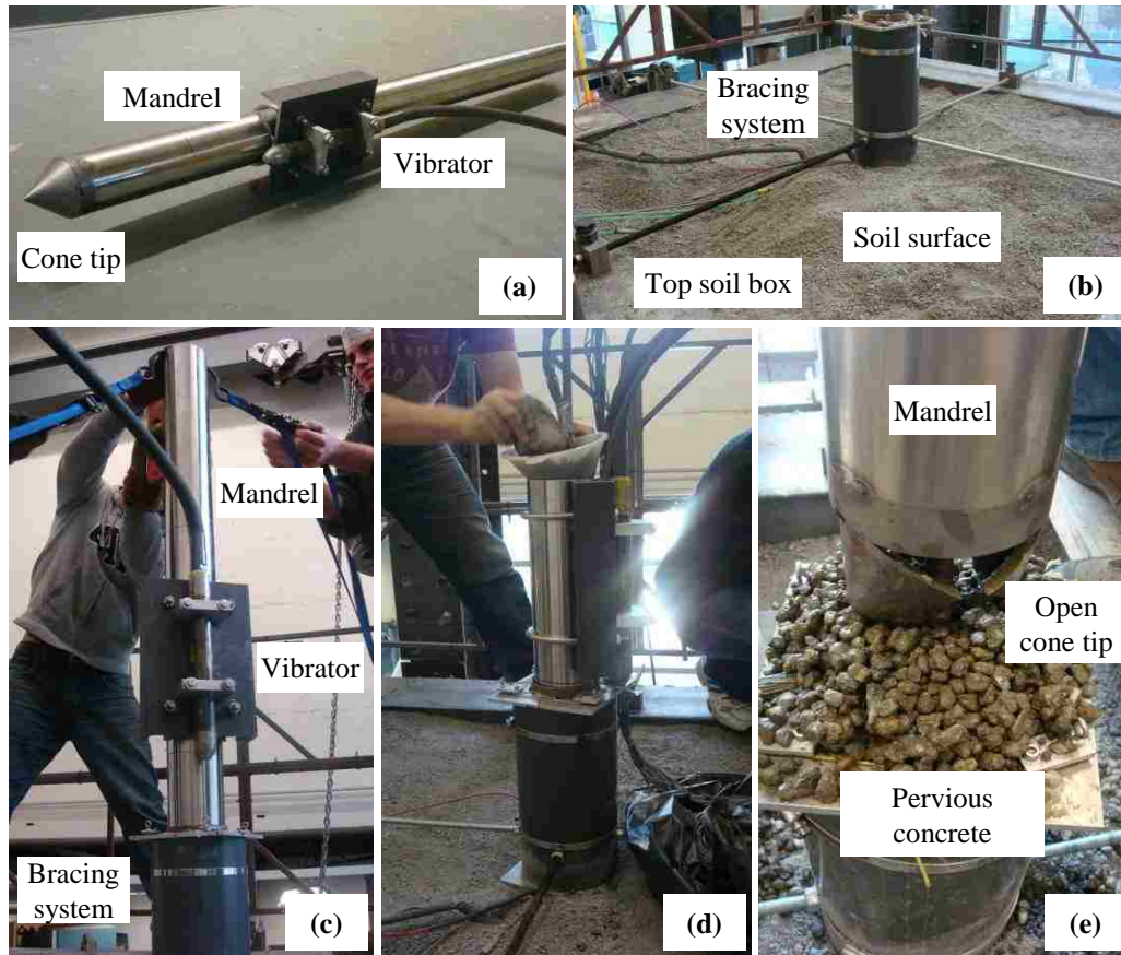
Figure 3.3 Summary of the developed pile installation method: (a) cone with vibrator, (b) bracing (guiding) system, (c) driving the mandrel, (d) casting the pile, (e) open cone during casting
